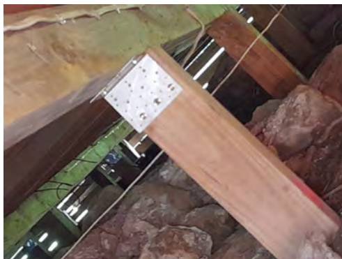
Example of anchor in wrong place.
